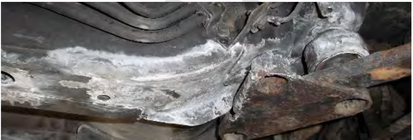
Image 3: very little iron oxide (rust) is neutralised/removed when acids are indiscriminately applied and not properly worked into the surface.
