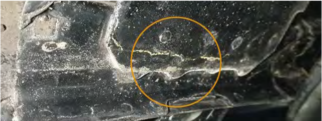
Image 6: acids not neutralised/removed (especially in difficult to access areas e.g. the inside of box sections and welded seams), can continue to attack any exposed metal surfaces, breaking down or degrading other protective coatings that they come in direct contact with, and allowing further corrosion to develop.
