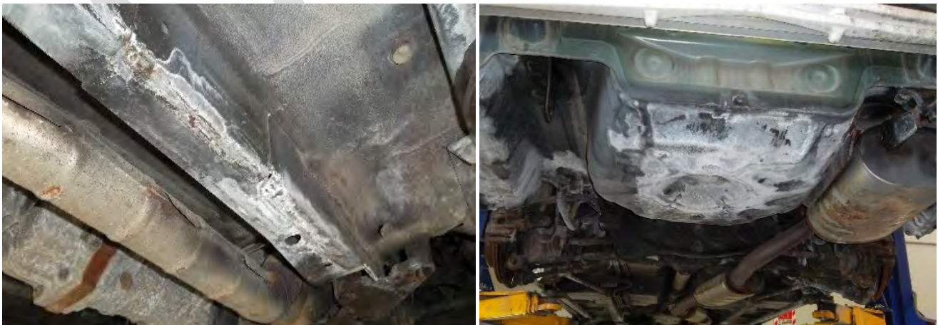
Images 4 and 5: the dry phosphorous coating created by the acid reaction to the metal (the white, powdery coating seen on the surface), is detrimental to the adhesion of subsequent topcoats.
