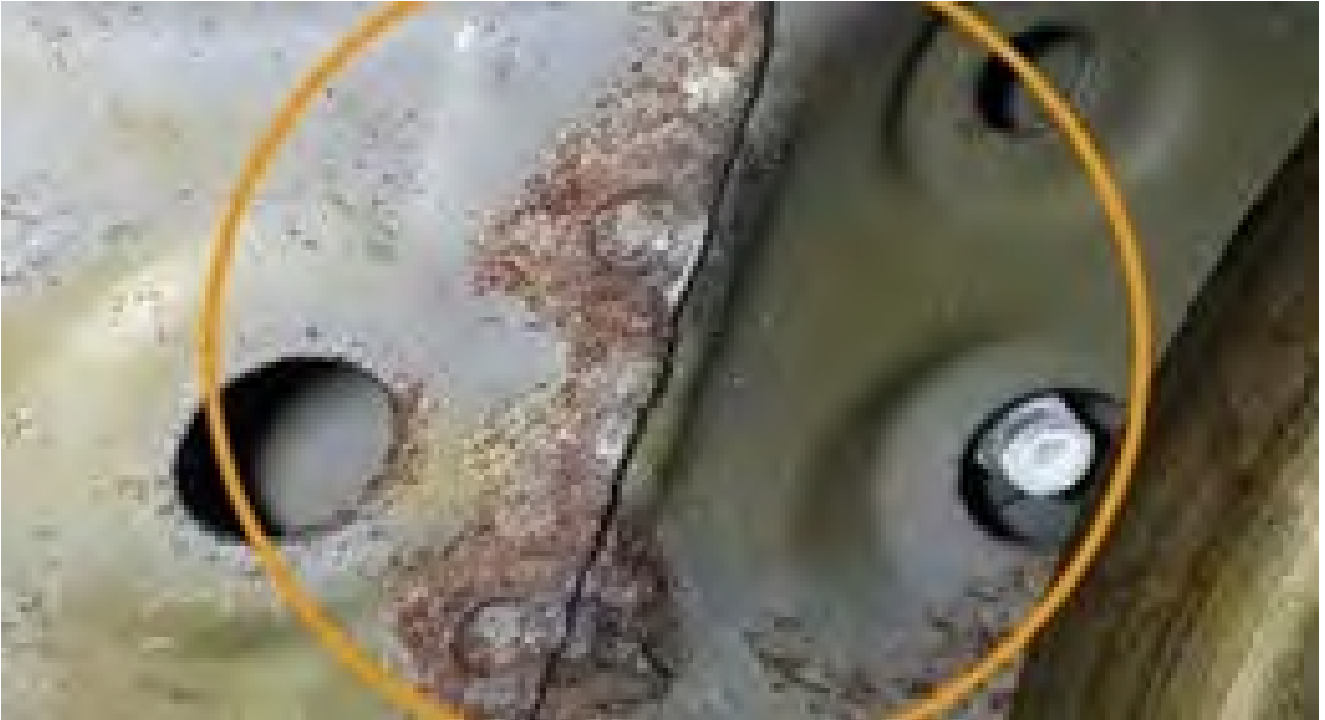
Image 2: loose/flaking rust scale has not been removed and is still present.
