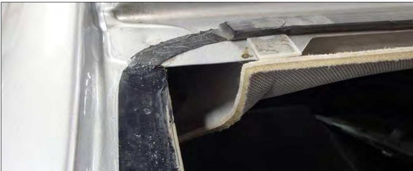
Image 7: Pinchweld flange Inspection and Preparation. Close-cut the original urethane down to a thickness of 1 mm - 2 mm. Clean with water and dry with a clean cloth.
